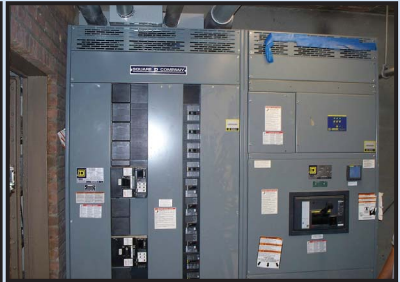
Replacement Electrical Distribution System
